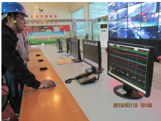
Processing Control Room
