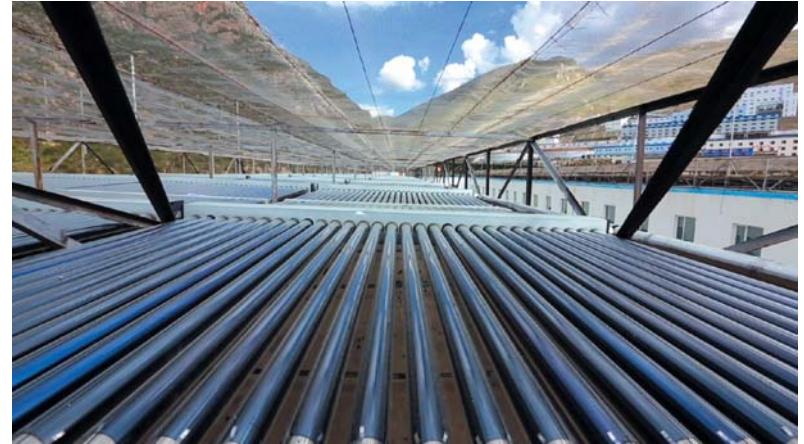
Solar heating equipment
