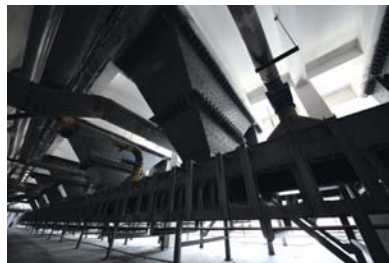
Hop-pocket dust catcher applied in the crushing plant
