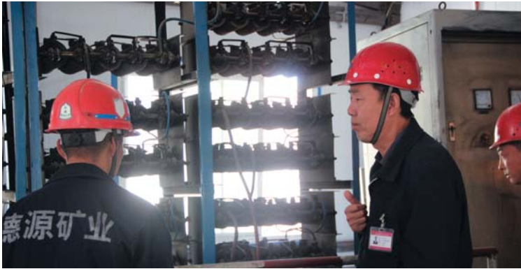
Safety supervision team inspecting electromechanical area in hoisting room of inclined shaft
